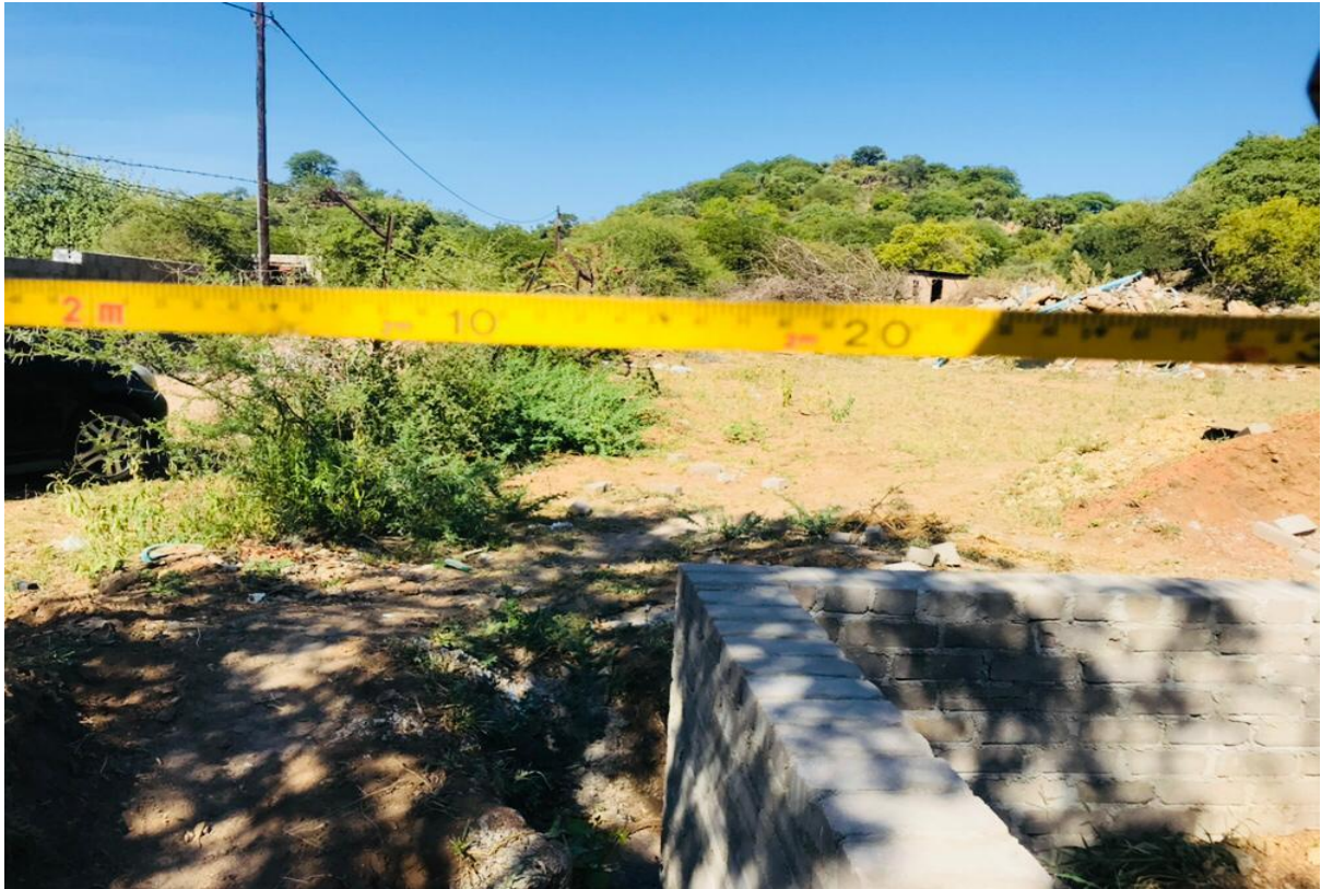
Picture showing the 2.2m width left between fence and the new structure constructed by PAP1 in 2019
